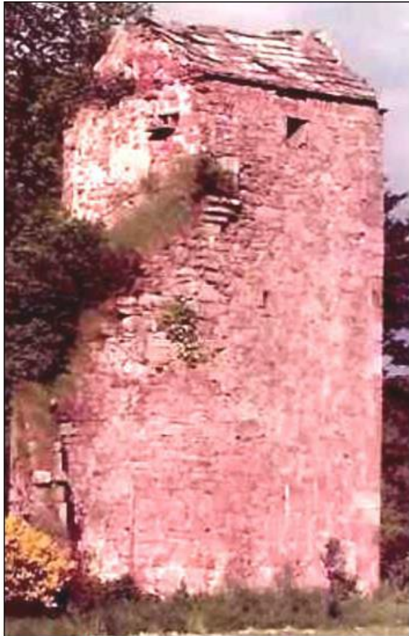
Blacket House as it appeared in the 1970s with the roof still intact.
